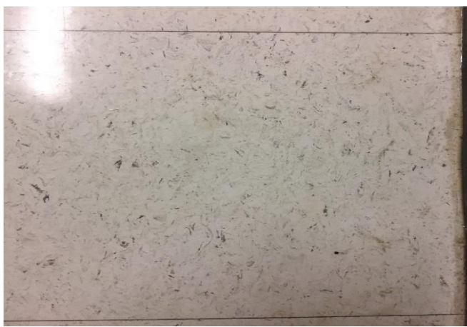
PHOTO 24 Asbestos containing 12"x12" vinyl floor tile, white with black streaks (2% Chrysotile); with asbestos containing black mastic (5% Chrysotile). HM#: MM-03/A ACM
