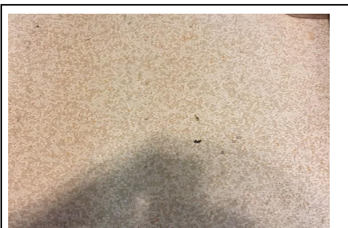
PHOTO 35 Asbestos containing sheet vinyl flooring (22% Chrysotile). HM#: MM-14 ACM
