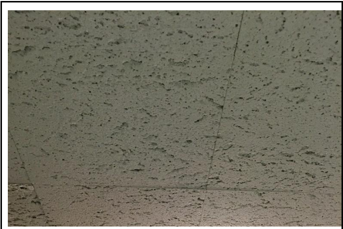
PHOTO 27 Non-asbestos containing ceiling tile. HM#: MM-06
