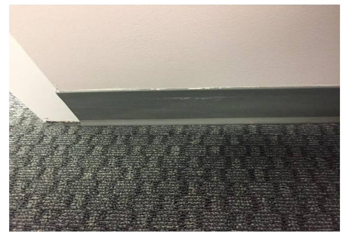
PHOTO 25 Non-asbestos containing 4" vinyl base. HM#: MM-04
