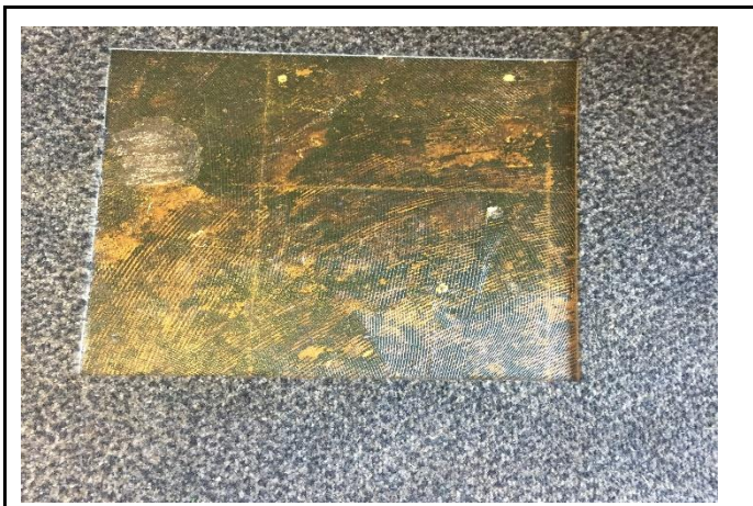
PHOTO 32 Asbestos containing black mastic (2% Chrysotile), underneath carpet squares. HM#: MM-11 ACM
